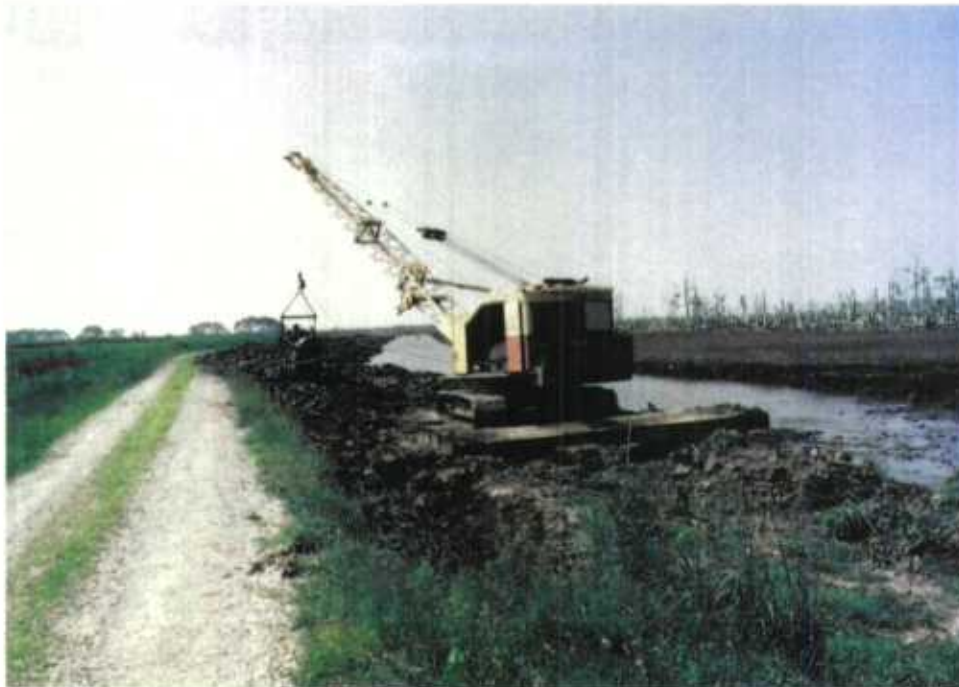
A contract dragline worked to re-core the inside shoulder of the Long Dike and add six feet of width to the dike. 5/93 BN
