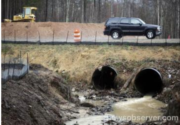
Figure 4-6 Perched culvert (credit: Raleigh News and Observer)
