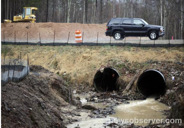
Figure 4-6 Perched culvert (credit: Raleigh News and Observer)
