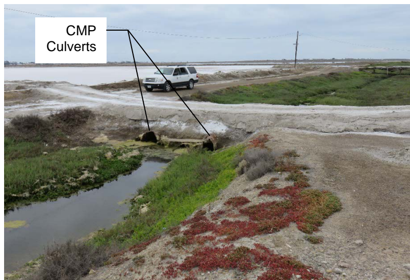
Figure 15. Existing CMP Culverts Providing Hydraulic Connectivity at the Channel Crossing Located North of Pond 30
