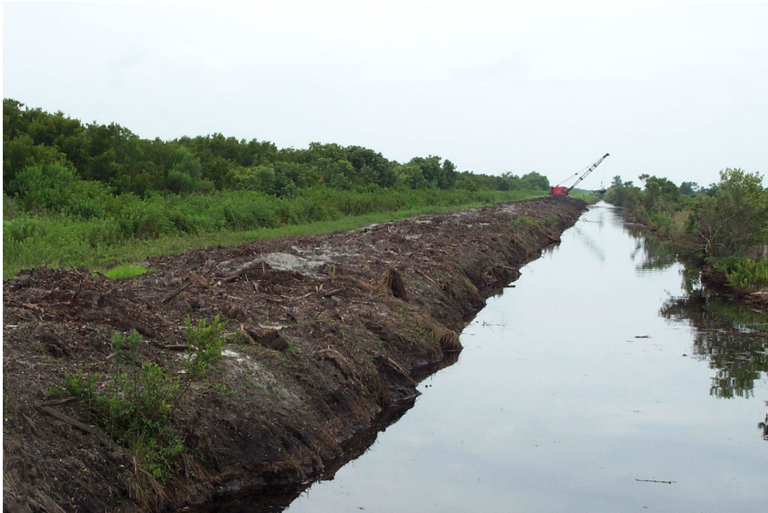
Figure A-10. Canal maintenance with excavated material placed on top of adjacent dike.
