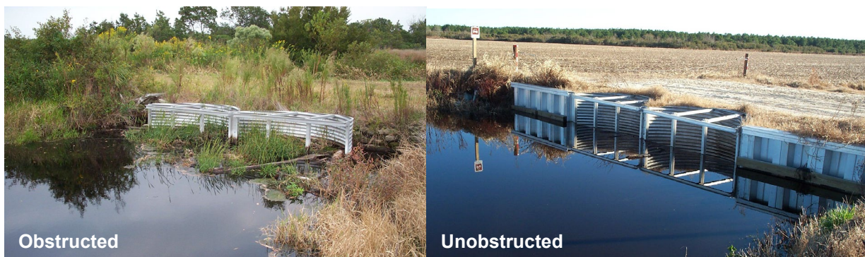
Figure A-15. Obstructed and unobstructed riser water control structures.
