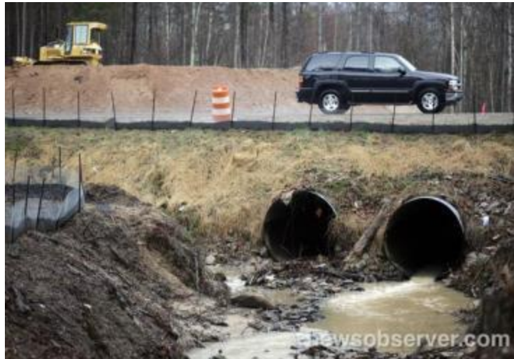
Figure 4-6 Perched culvert (credit: Raleigh News and Observer)
