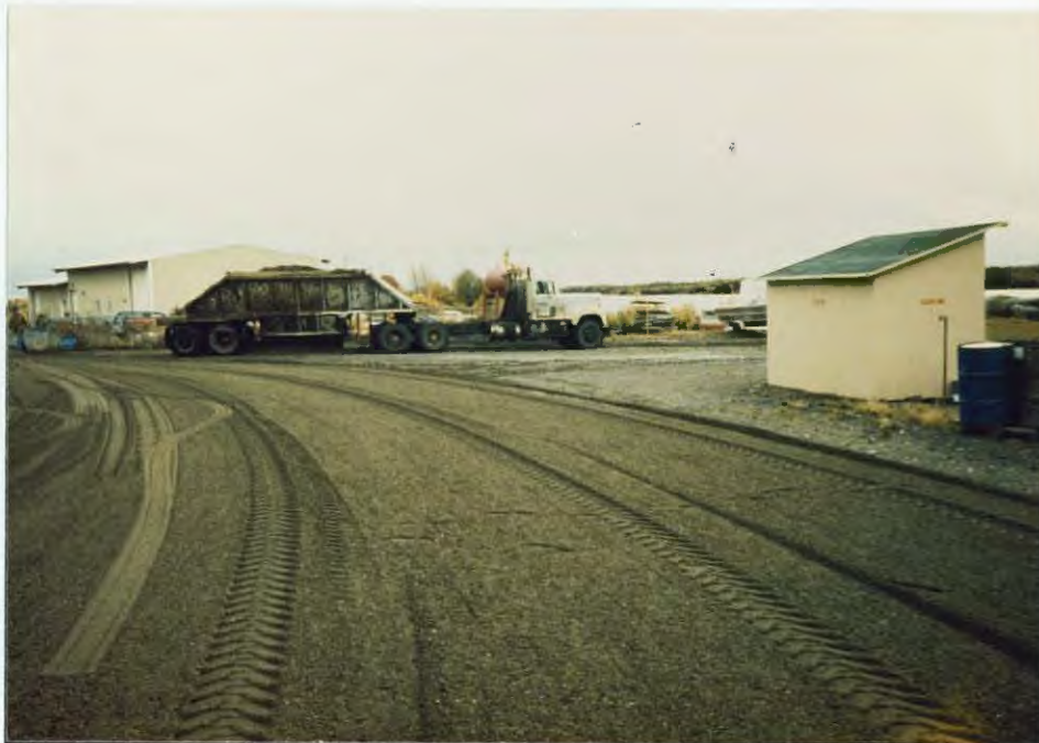
Gravel truck delivering part of the 325 cubic yards of gravel for the headquarters parking area.
