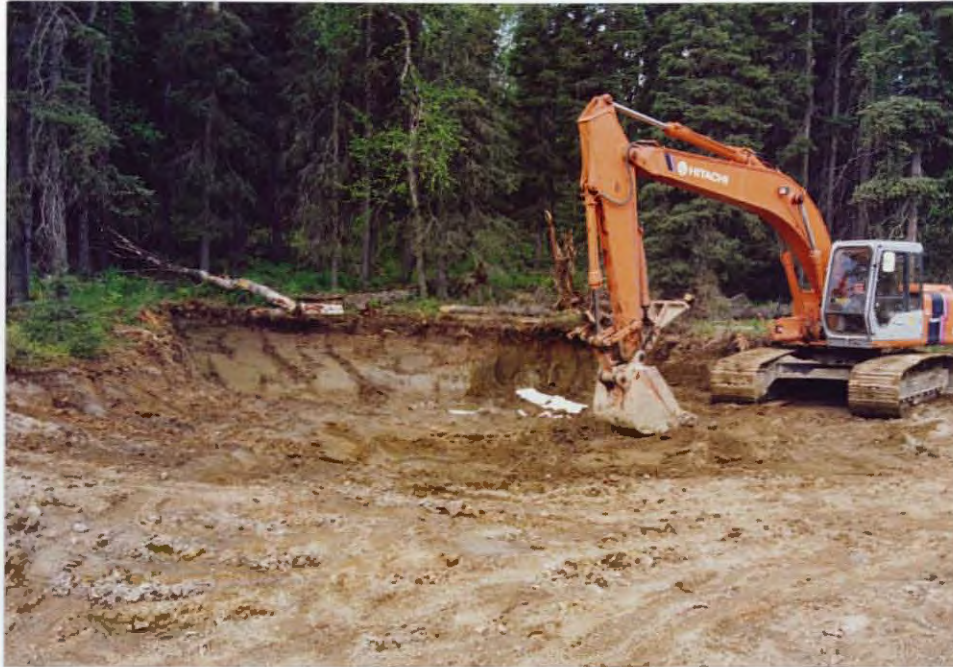
Excavation for contaminated soils following break in the 2-15 crude transfer drain line. 92/JF
