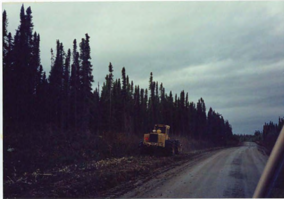
Approximately 20 miles of roadside along the Swan Lake/Swanson River Roads were hydro-axed by Operator Kivi. 92/JF
