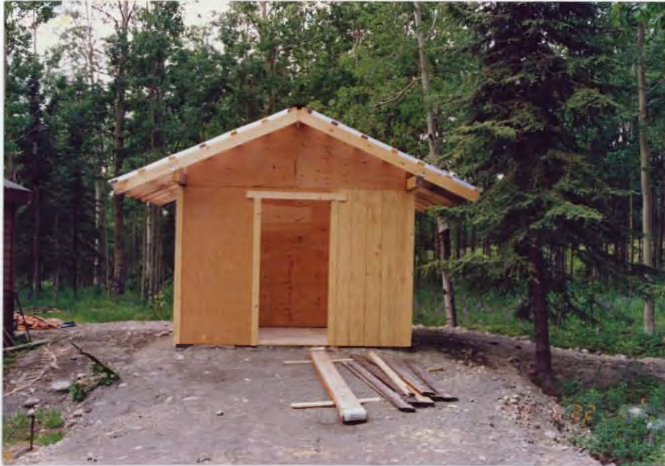
New generator shed constructed at the Skilak Guard Station will house a new 5KW diesel generator to meet the facility's electrical needs. 92/JF
