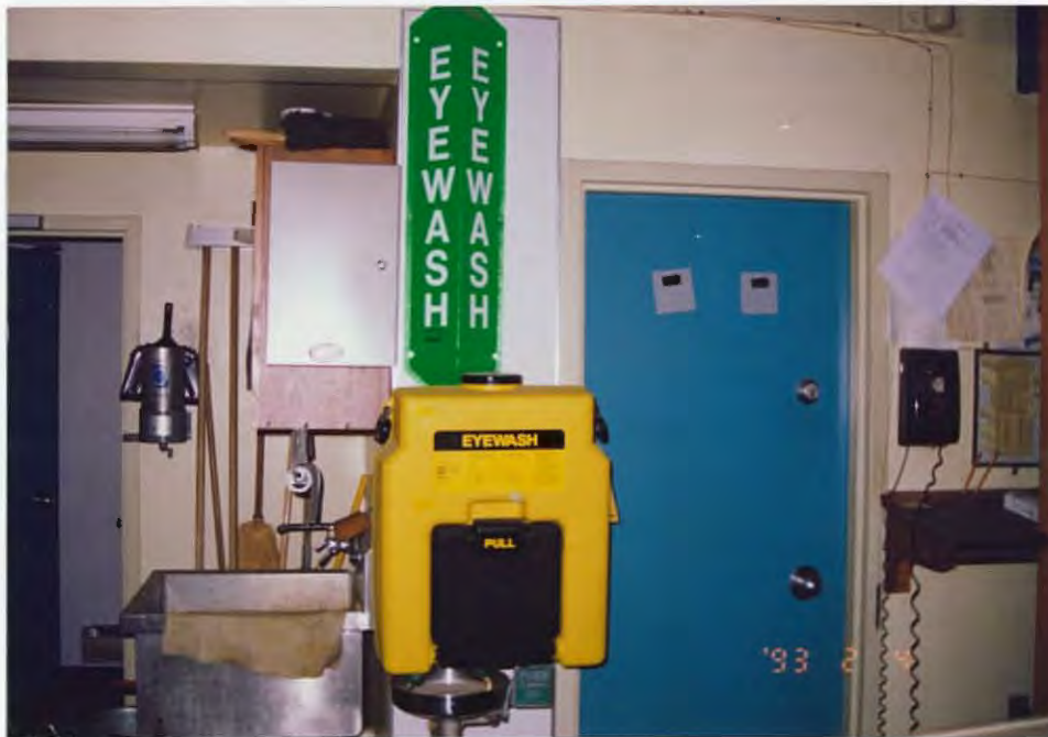
One of two new emergency eye wash stations installed at maintenance shop. 92/JF
