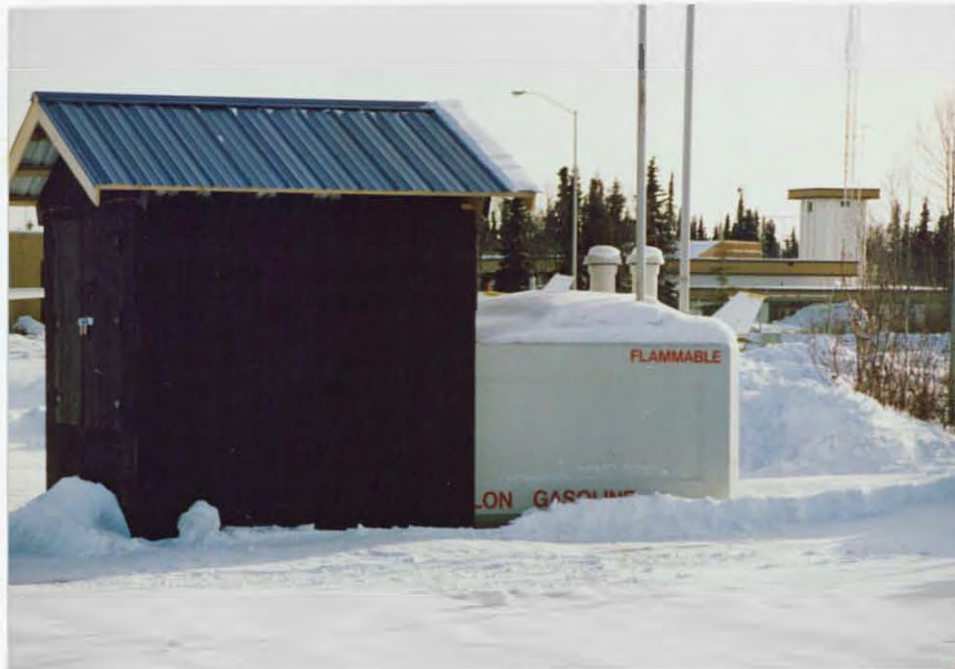
An all-weather shed was constructed to protect the hose, reel, pump, and meter at the new Kenai Hangar aviation refueling facility.
