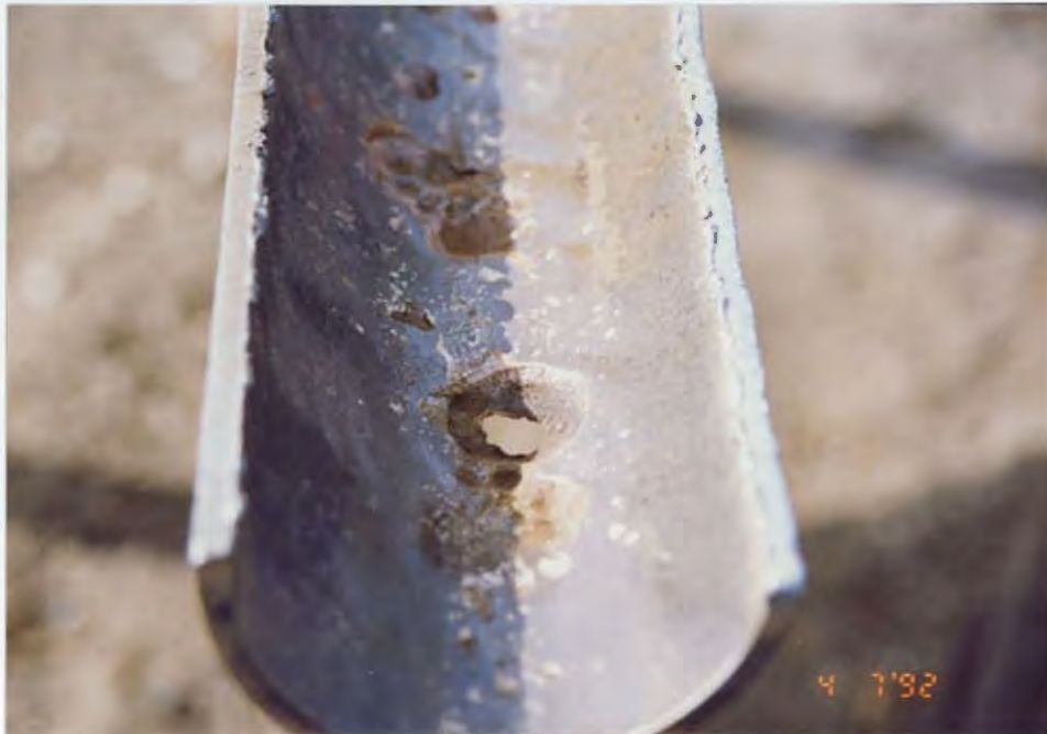
Severe corrosion in the 2-15 drain line prompted an extensive effort to determine the integrity characteristics of other long-buried lines within the field. 92/JF
