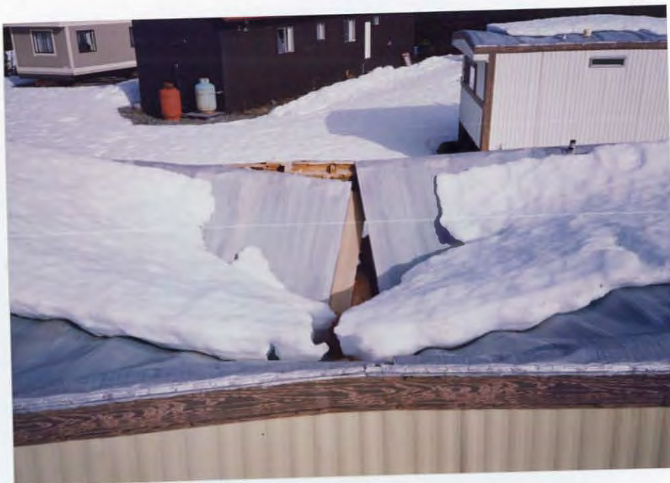
Near-record snowfall during the winter of 1991-1992 proved too much for the fragile roofs of trailers at Schooner Bend Field Camp. 92/JF
