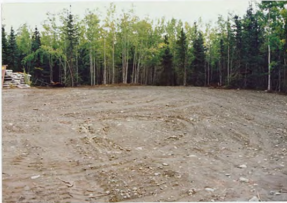
Skilak Guard Station drum storage/bone yard following excavation and leveling of contaminated soils. 92/JF
