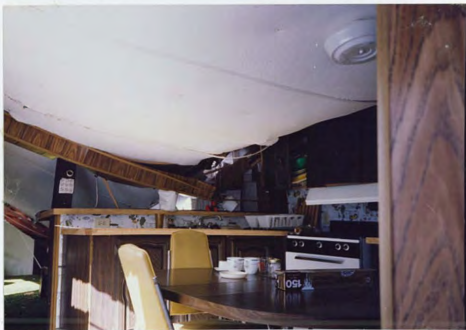
Interior damage from collapsed roof of 14' X 60' trailer at Schooner Bend Field Camp. 92/JF
