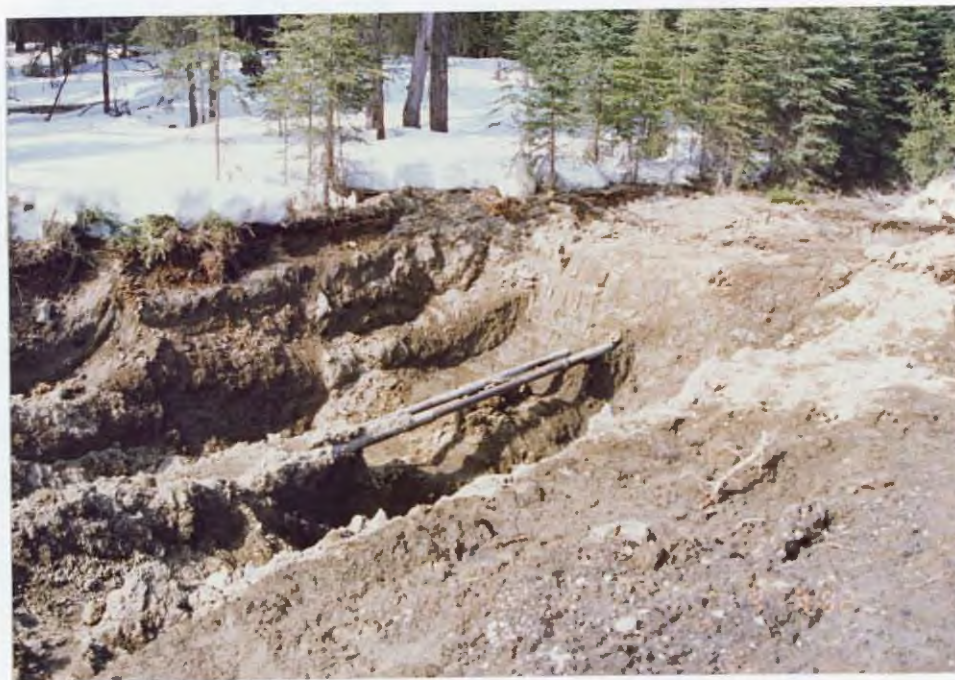
A leak in the 2-15 drain line was the source of a major crude spill within the field in March. 92/JF
