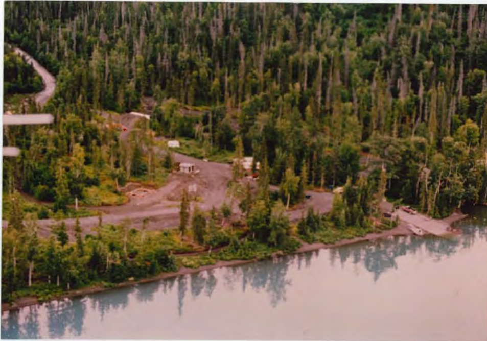
Upper Skilak Campground construction gets underway with a newly completed boat ramp, gravel road bed construction, and new toilets, 1992. Unknown
