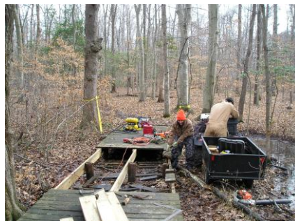
Woodmarsh Trail boardwalk before repair
