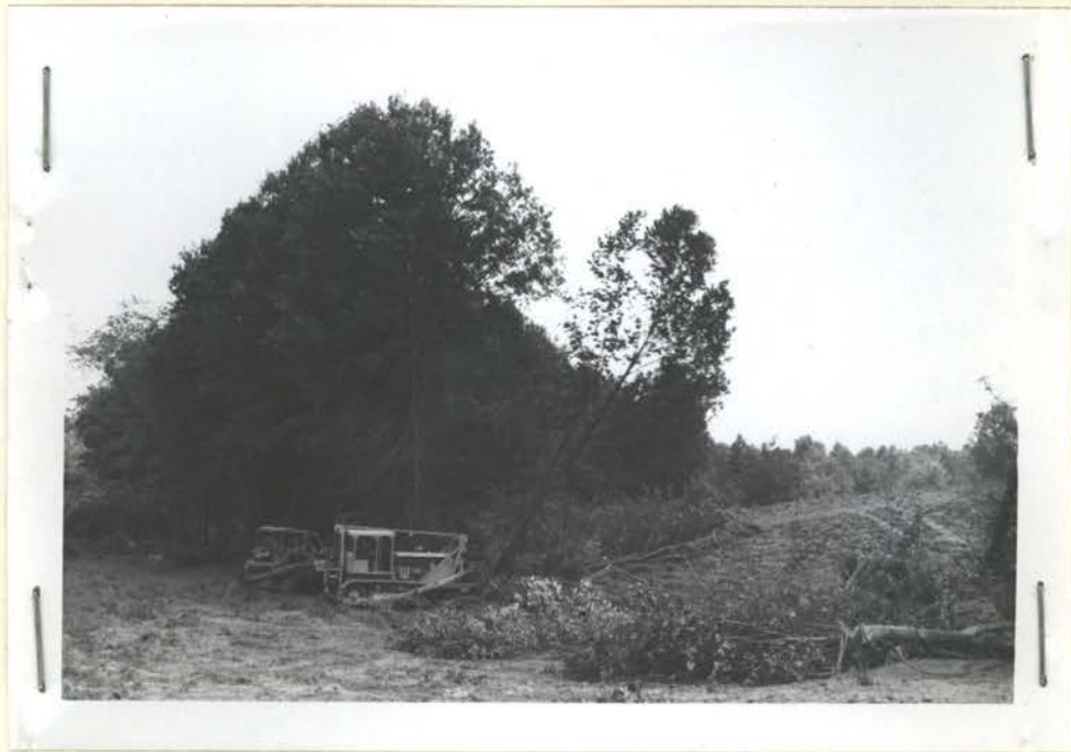
Over 200 acres of brush and timberland were cleared for pasture development. The D-8, in action here, can handle most of the big stuff. The D-7 and TD-14 take care of the rest. A large root rake would make this combination perfect. R-9-1. 7-60, Carter.
