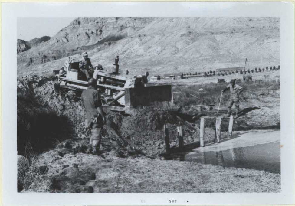
Above: Dirt is pushed against wooden structure to build a jetty on which to place pumps. Now if it will just hold .....
