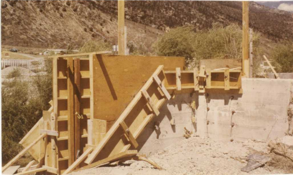
The $92,000 BLHP project for repair of water control structures was left incomplete at years' end. This structure behind Gallagher Hatchery was the only one completed. MDS 8/79
