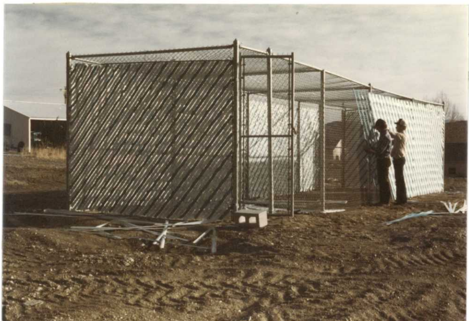
Refuge and YACC personnel began constructing a new raptor rehabilitation facility in September. FWC 9/79
