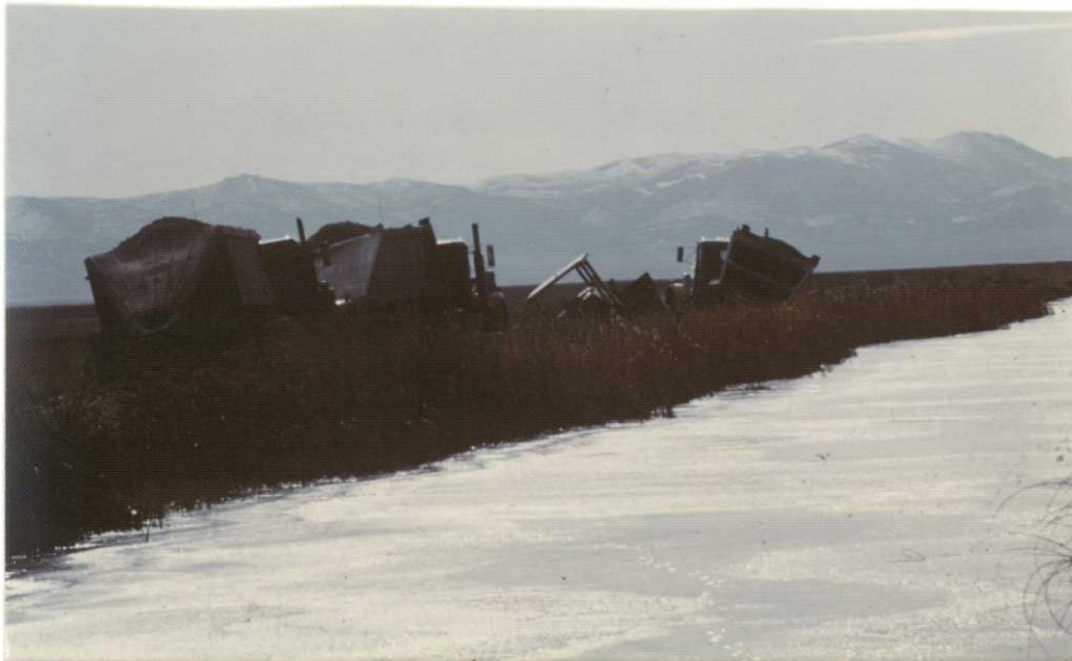
The BLHP dike resurfacing project had several delays including this mired mass of equipment. The $38,134 job was completed in May 1979.
