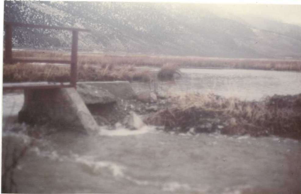
The area to the right of this structure into Unit 21 has been washed away. The photo was taken after water had receded about two feet.
