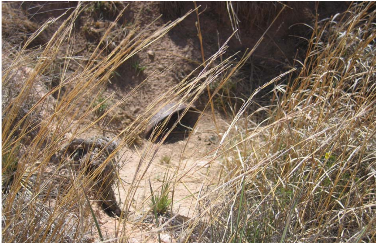
Photo #878 - MP 0.00 – Drainage deficiency
