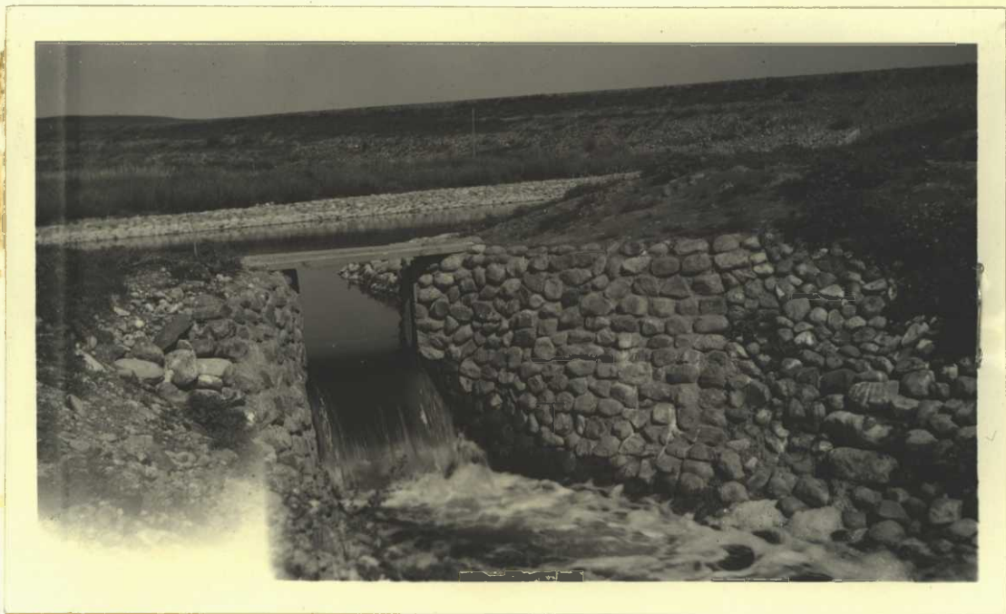
The flashboard control below Dam 83.
