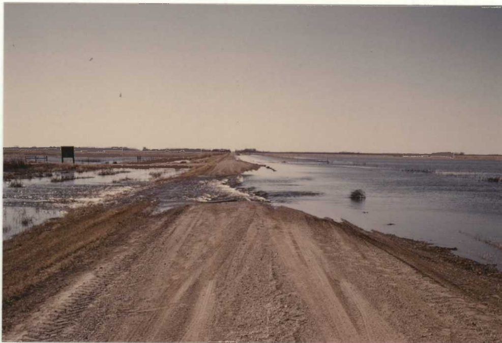
Photo # 1. Water rushing from the upper watershed overtopped the Maza-Garske road on the north side of the refuge. 4/87 DAL
