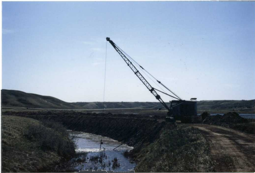
GERALD FELCH CLEANING OUT UNIT 7 BY-PASS DITCH. NOTE: EMERGENT VEGETATION IN DITCH PRIOR TO CLEANOUT.
