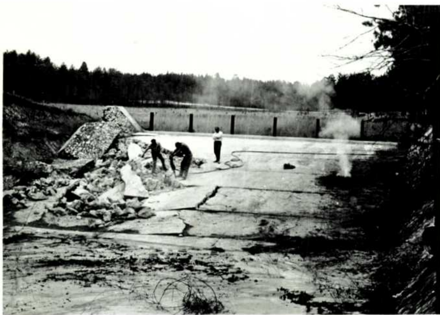
A flash flood in 1957 washed out the spillway of 14 acre Lake Bee. As a part of the forest recreation phase of the Accelerated Public Works program begun in 1963, the spillway was renovated in mid-summer of 1964. No. 14
