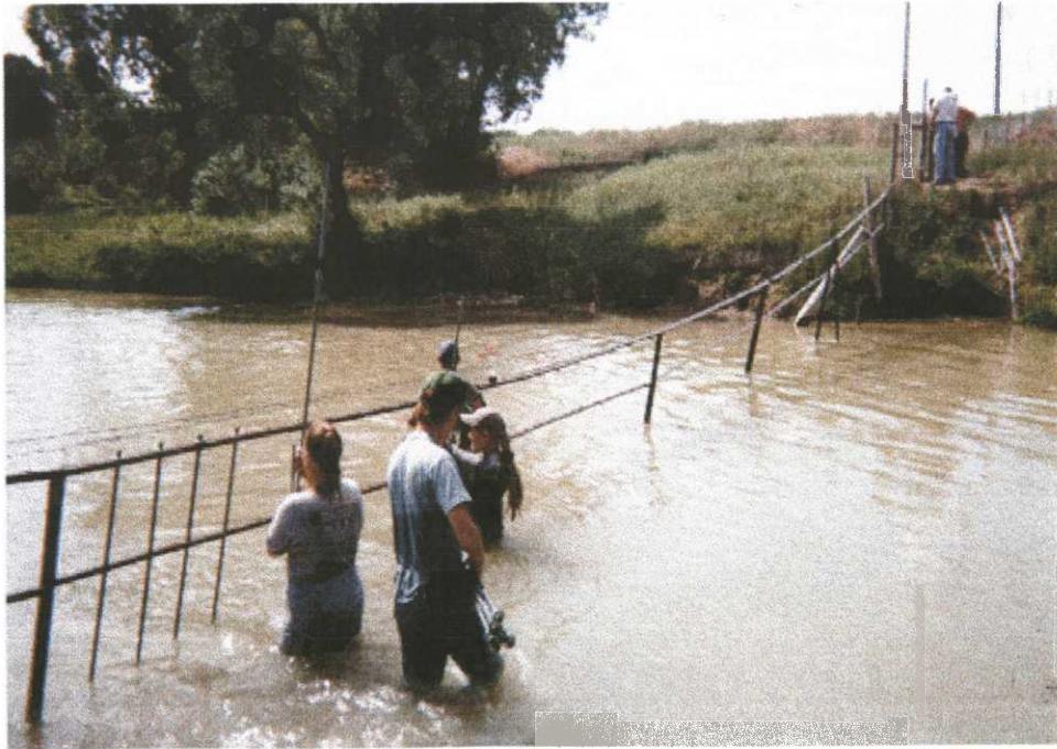
Figure 2. YCC designed and constructed a boundary "fence" across the fluctuating Lake Alice outlet that will permit debris to flow downstream yet keep cattle out.
