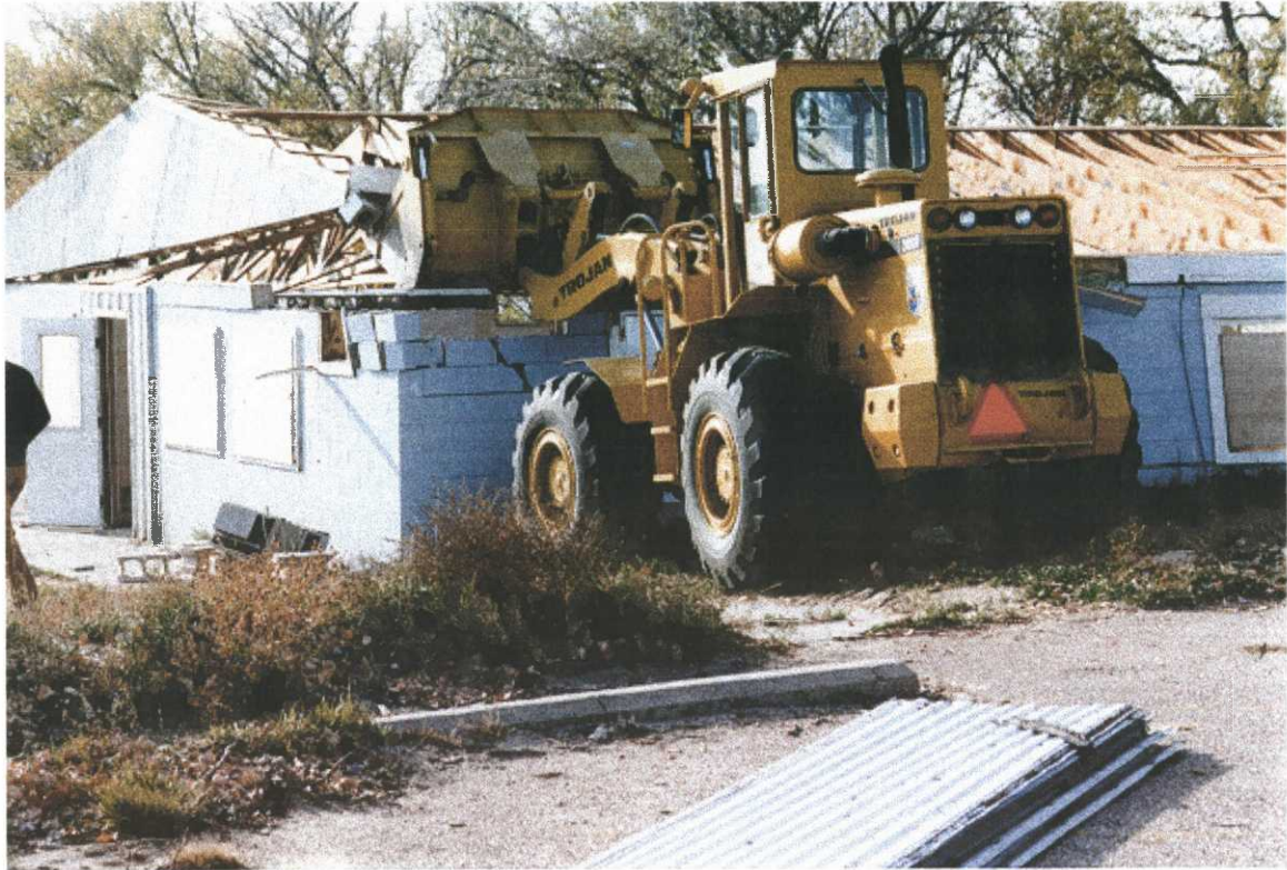
Figure 9. The former concession building was razed following contractual removal of asbestos. NGPC is considering building a visitor center on the site and has asked the Project Leader for means of securing Service contributions for shared space in the new facility. 96NPL9-BWM
