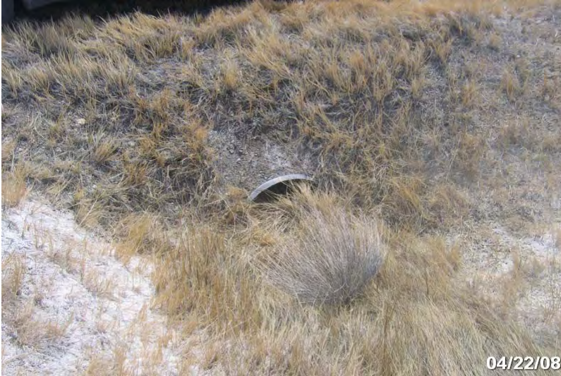
Photo # 3853 - MP 0.07 - Culvert Deficiency
