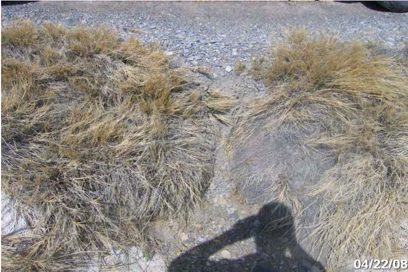
Photo # 3854 - MP 0.07 - Culvert Deficiency
