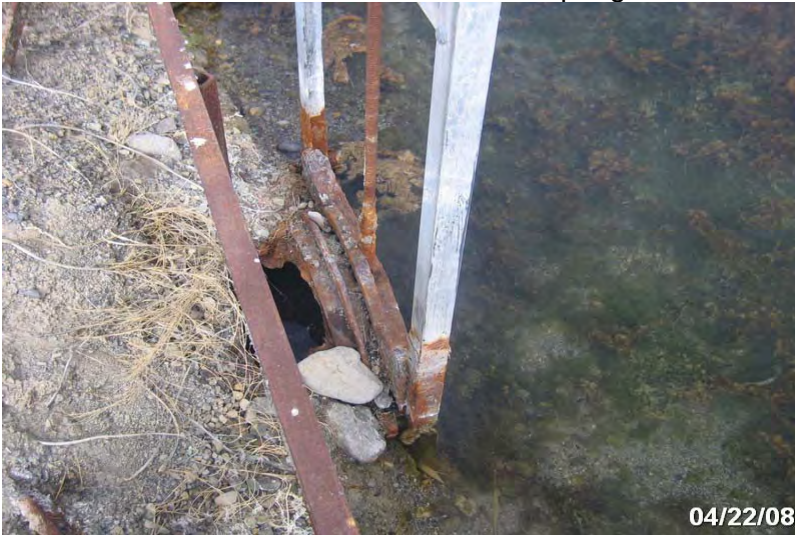
Photo # 3807 - MP 0.62 - Culvert Deficiency
