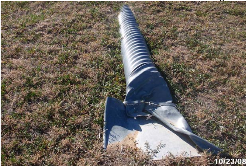
Photo # 2087 - MP 0.15 - Culvert Deficiency
