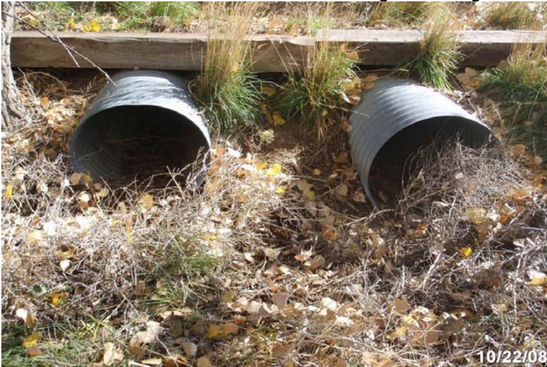
Photo # 1998 - MP 0.67 - Culvert Deficiency
