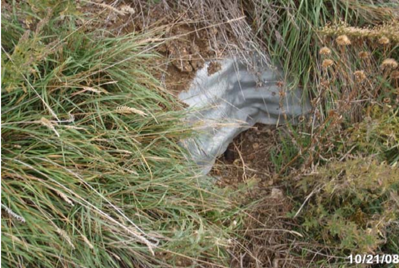
Photo # 1903 - MP 0.75 - Culvert Deficiency
