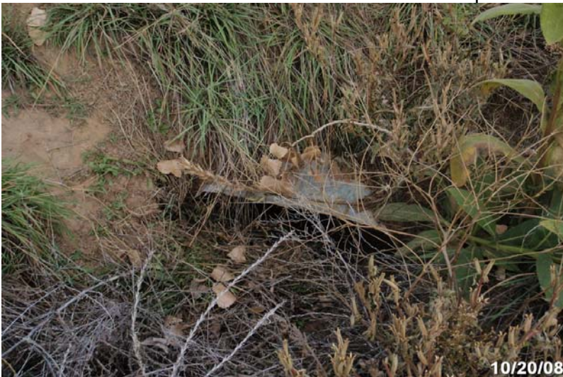
Photo # 1853 - MP 0.01 - Culvert Deficiency
