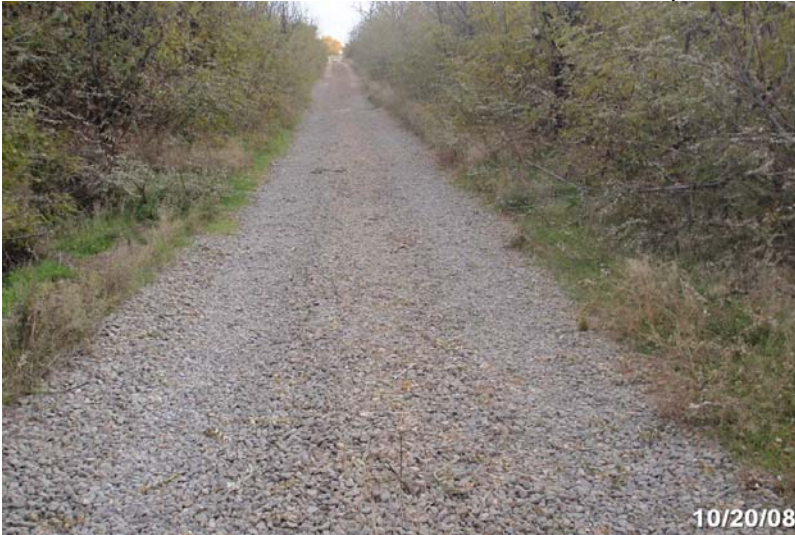
Photo # 1854 - MP 0.01 - Culvert Deficiency
