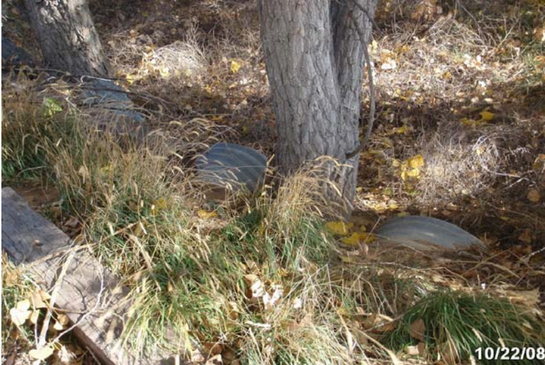
Photo # 1997 - MP 0.67 - Culvert Deficiency
