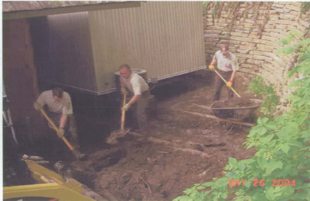
Mud cleanup behind the office building and office trailer.
