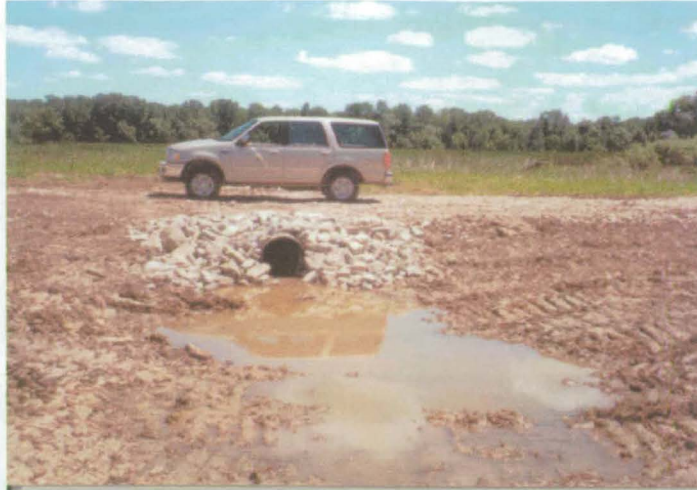
New culvert between North Marsh and Eagle Marsh will improve fish passage during spawning season. (EPD 7/2000)
