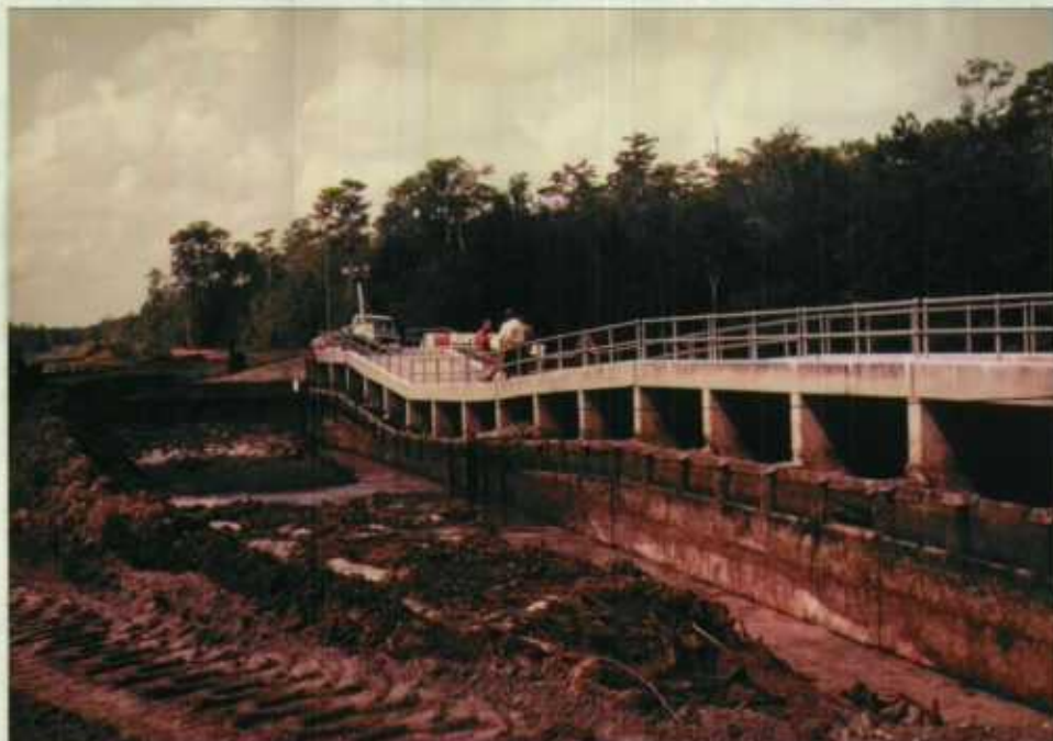
Damaged Suwannee River Sill Water Control Structure. (TW) 5-OKE-79
