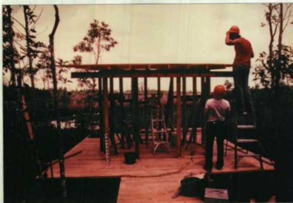
Refuge work on the boardwalk spur. (December, 1978) (Job Order No. 2821-897-T4) (TW) 53-OKE-79
