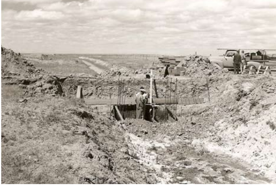
Figure 19. Construction of levees and water-control structures on Benton Lake National Wildlife Refuge in 1960.
