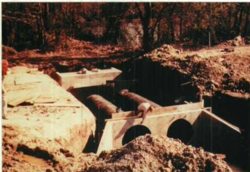
This new control structure was completed and functioning before the end of the year.
