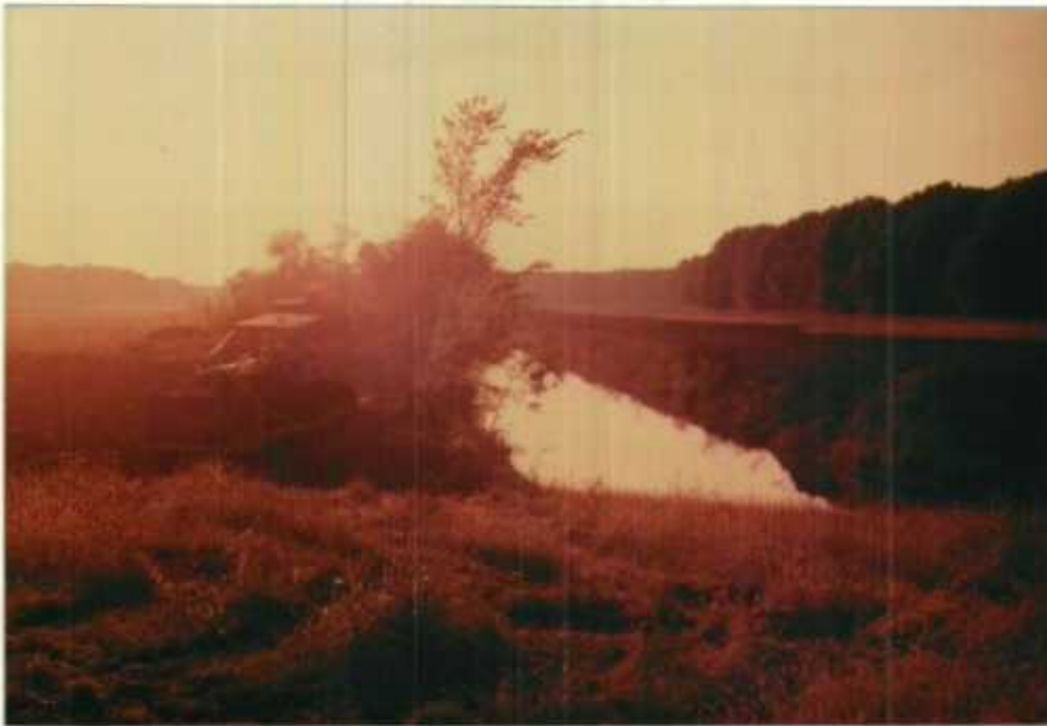
Spoil piles were leveled after the cleanout of the dewatered ditch system was completed.
