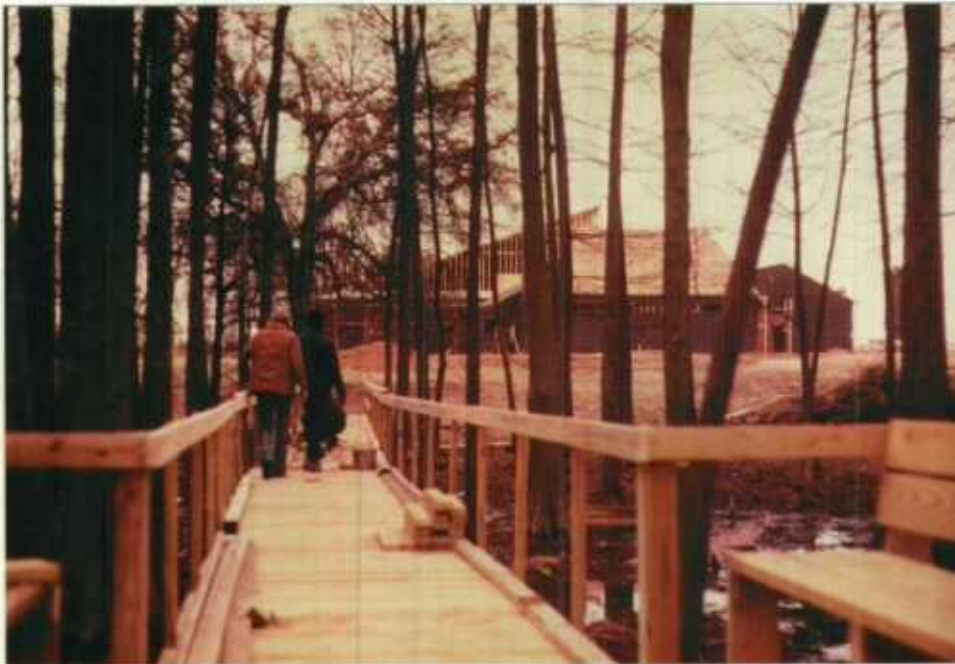
The Cypress Pond Boardwalk nearing completion. This structure was completed and stained during the year.
