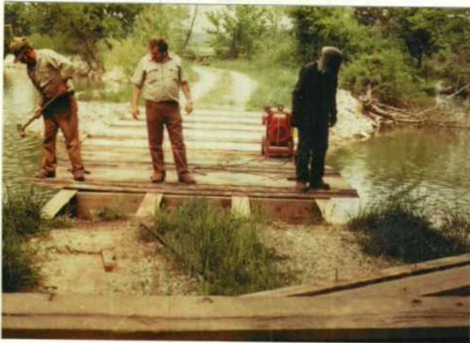
All refuge bridges are now all-steel construction. Photo shows employees steel-flooring Dinsmore Slough Bridge.
