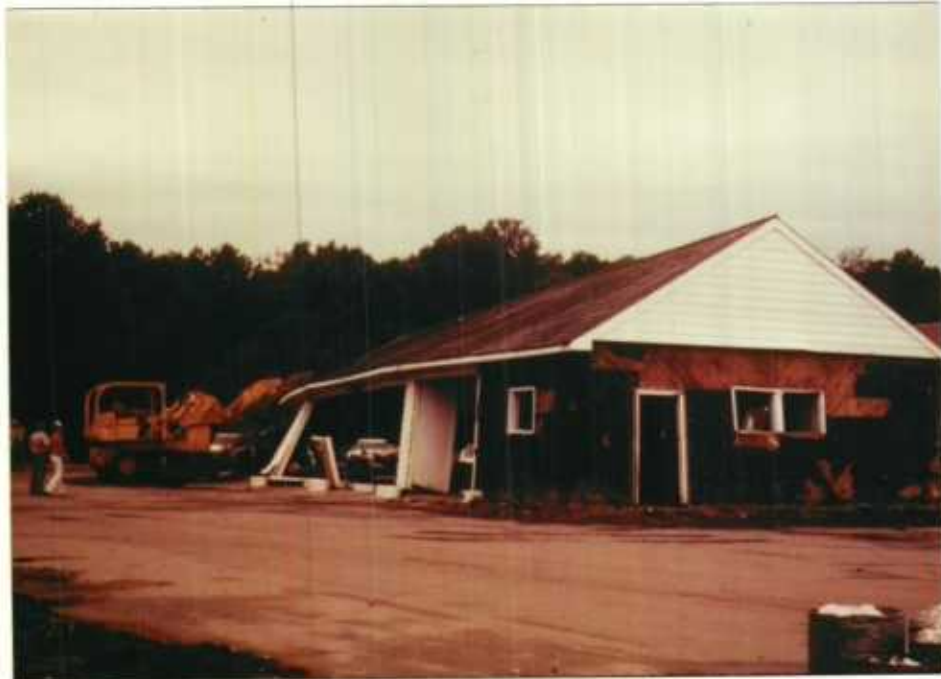
The old shop-garage building, in the way of construction, was demolished by forced account.
