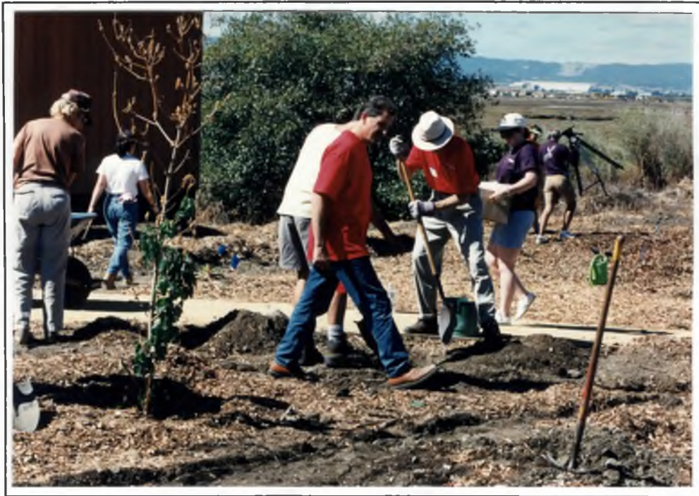
Volunteers from Viacom work hard to create a new Migratory Songbird Garden by installing drip irrigation and planting native plants around the P.O.S.T. pavilion.
