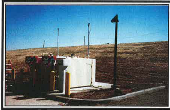
The gas pumps were installed with computer connections to monitor gas use for each driver and vehicle. They are programmed to “beep” when service is needed for the vehicle being fueled.
