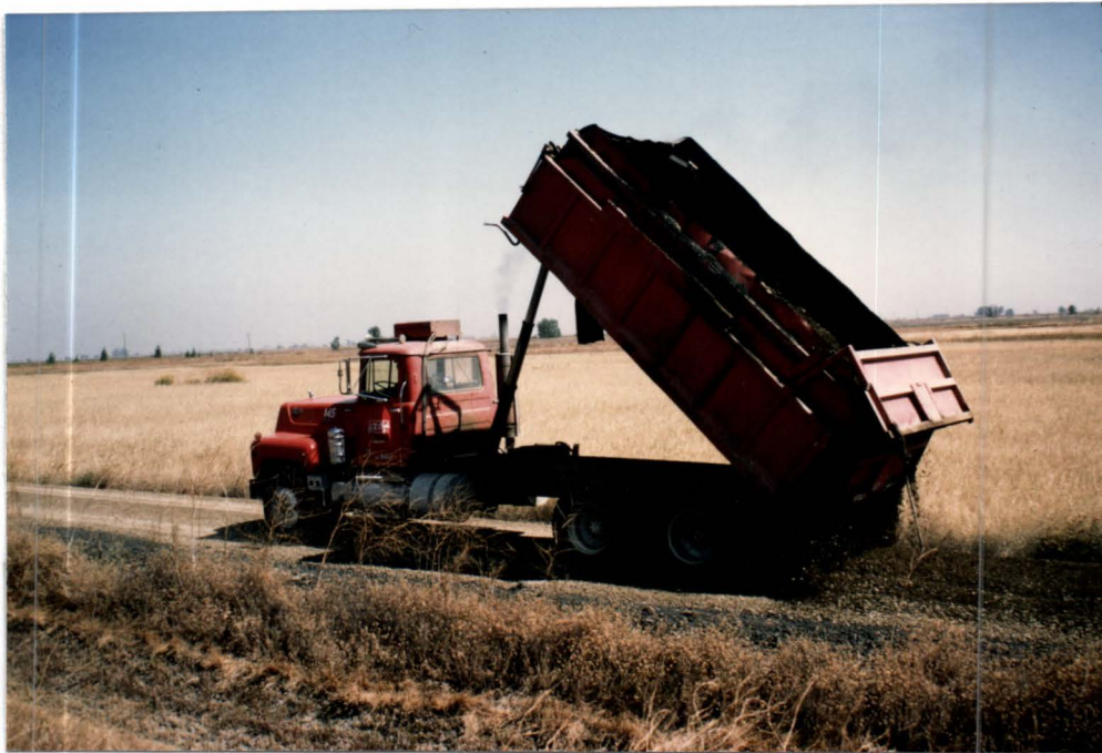
The pump 16 road was one of many roads which underwent extensive rehabilitation and graveling. 9/92 TJM
