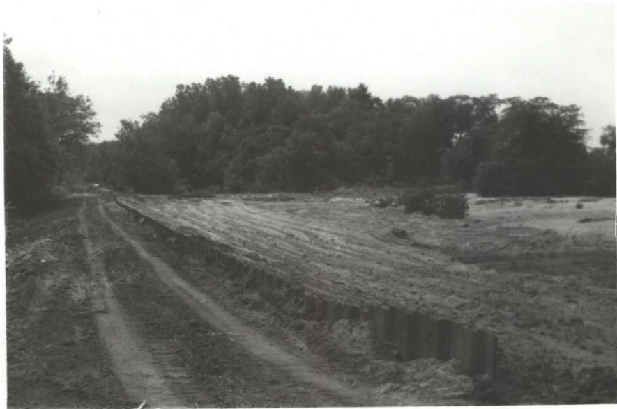
Eight foot lengths of sheet piling were driven into 10-15 feet of sand to prevent washing the outlet side of the spillway.
