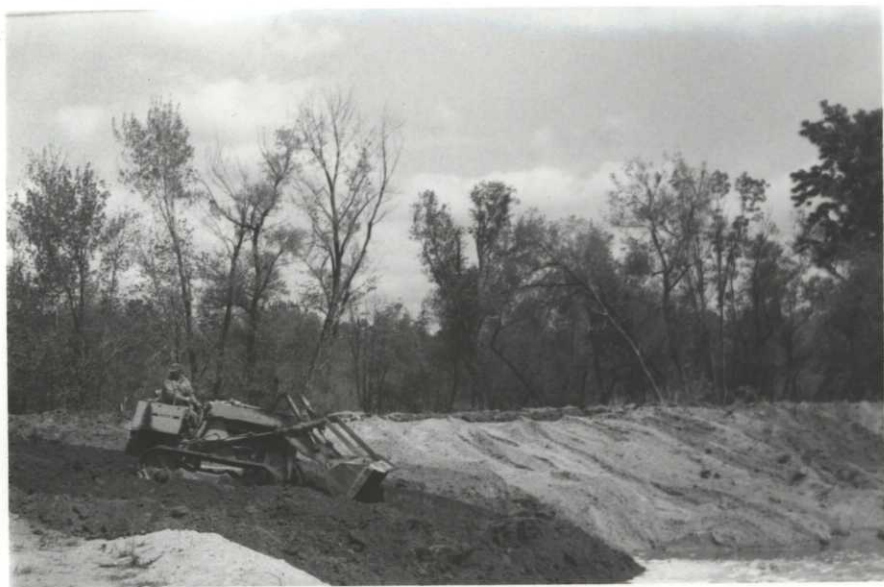
A contract was let in 1971 to construct a second spillway in the Keithsburg Levee.
