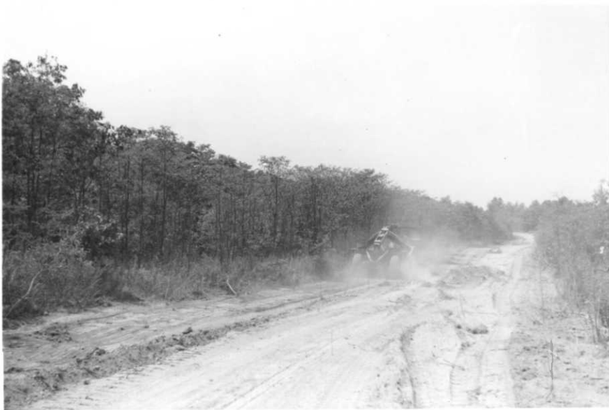
Dozer & scoop working on section of westside fire & timber access trail near Crump place
