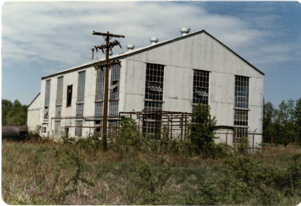
A-3 road boiler house before demolition. Area was returned to wildlife habitat.
