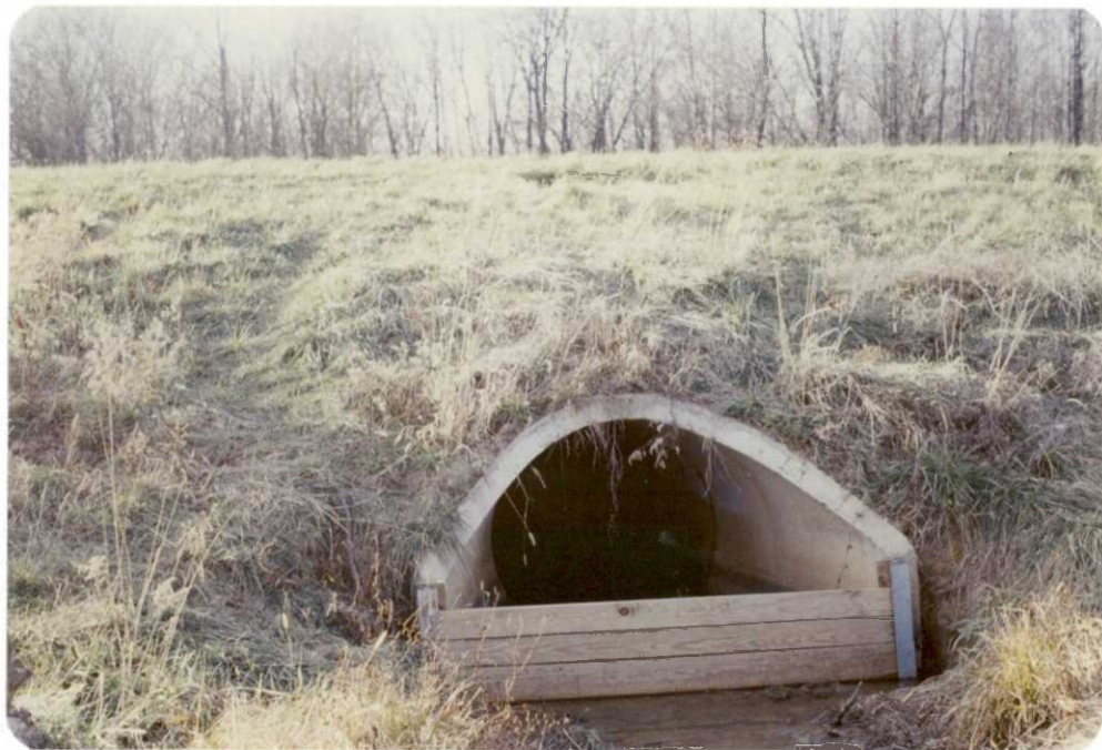
Stoplog structure on I-57 installed by state Highway department to re-flood 35-acre wetland.
